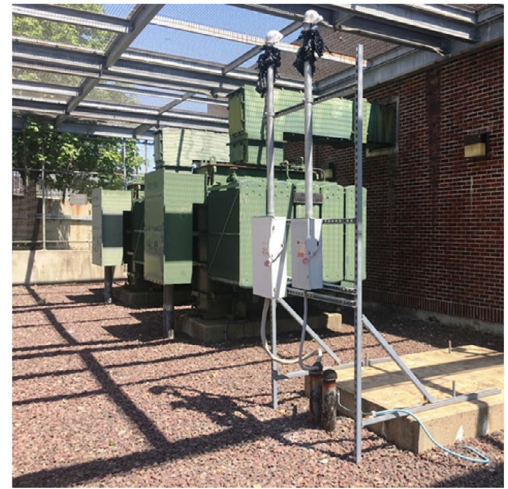
Figure 3-9 DC Traction Power Substation—Rectifier Transformers in Open-Air Enclosure
