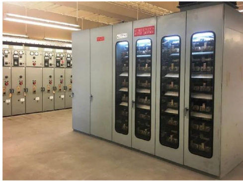
Figure 3-8 DC Traction Power Substation—Rectifier and Switchgear Equipment Inside Substation Housing
